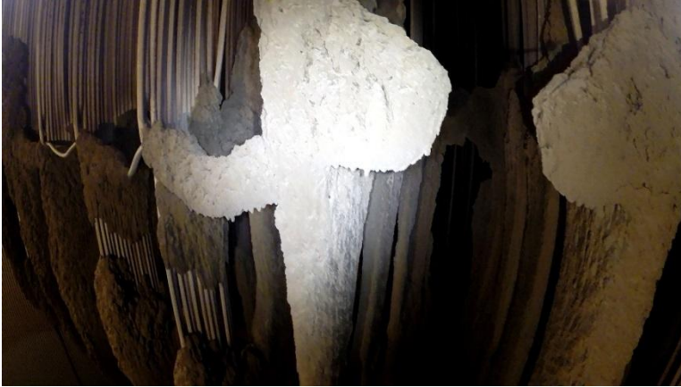
Figure 2. Plugging of pendant sections in a coal-fired boiler
