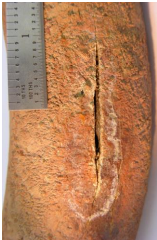
Figure 1. Thick slag build-up on a reheater tube after switching to PRB coal.
